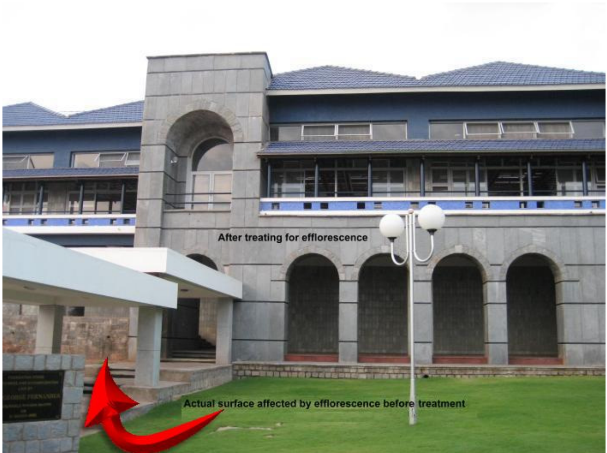
Before and after treatment of Efflorescence on unpolished S-white Granite slab and grout joints. After removal of efflorescence the surface has been treated with a wet look sealer.
